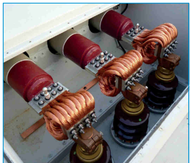
Copper braids to transformer
