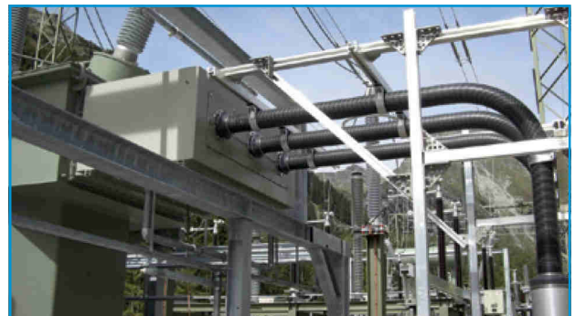
Switzerland - KW Löbbia: 17,5kV - 4000A
